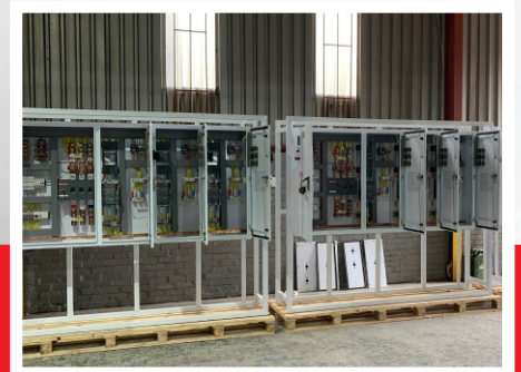
250kW Train Starter for Kamo Copper
