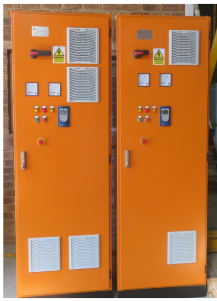
VSD Panel for Ore Crusher WEG
