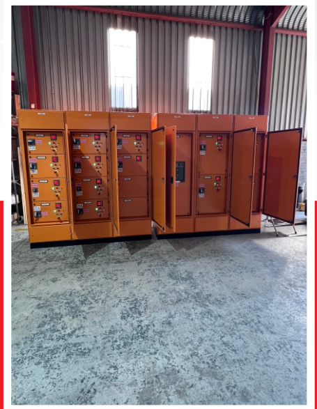
2000A Motor Control Centre for a customer in Africa
